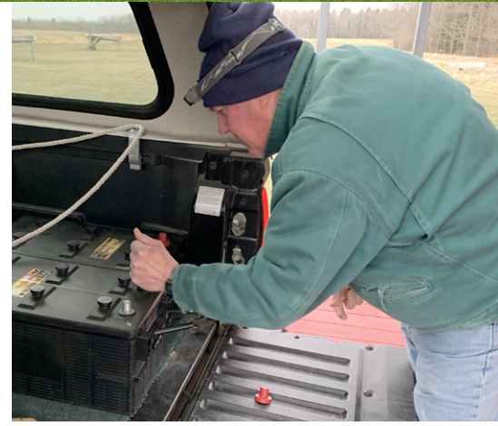
Elliott cleans the terminals of the new batteries before installation to assure a good connection.
